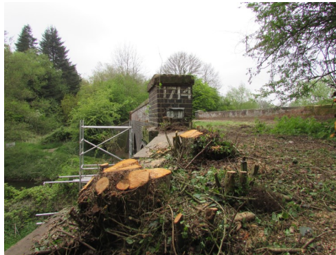
Removal of vegetation and damaging trees from bridge 1714 over the river Wensum.
