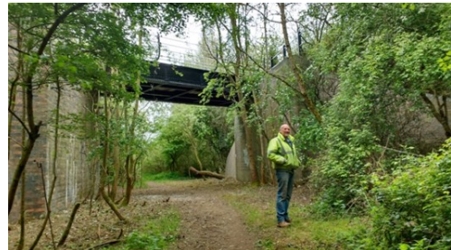
Paul Clifton on the M & G N track bed in front of repaired bridge 1715.
