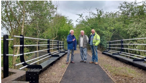
Trustees Trevor Bailey and David Bill with Greenford Ltd. foreman Paul Clifton on the repaired bridge 1715.
