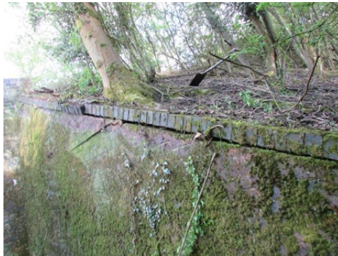
Masonry damage to bridge 1714 before repairs.
